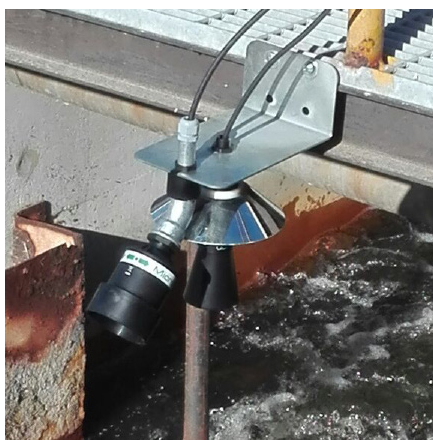
MicroFlow and dBMACH3 in a wastewater application
