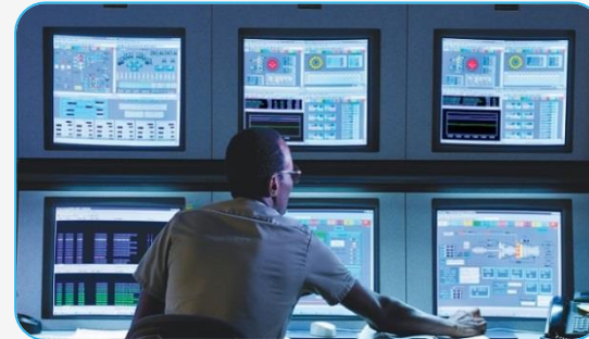
Building Management System
